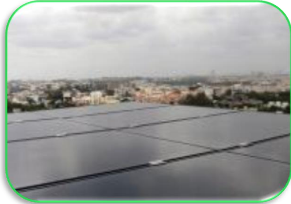
High Efficiency roof top solar power plant at Silicon House of Nava Limited.
