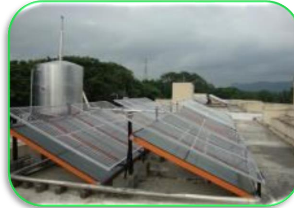
Solar water heaters at guest house and Bachelor hostel at Dhenkanal & Paloncha
