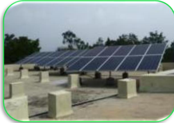
40 kW Solar Power Unit installed at Nava Bharat Schools, Paloncha
