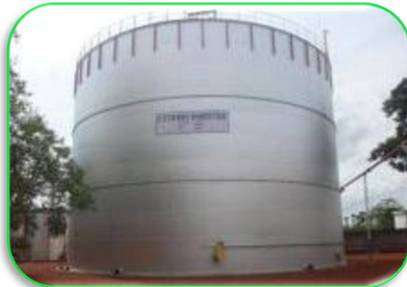
Installation of CSTR Bio-Digester to recover biogas and to use the same as fuel to distillery boiler.
