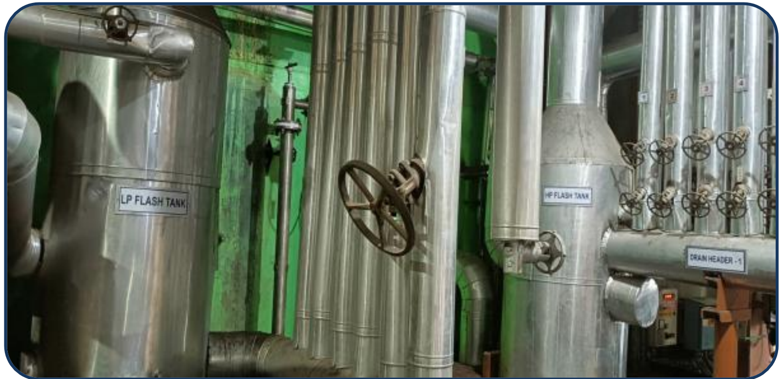
Dedicated LP & HP Flash tanks
