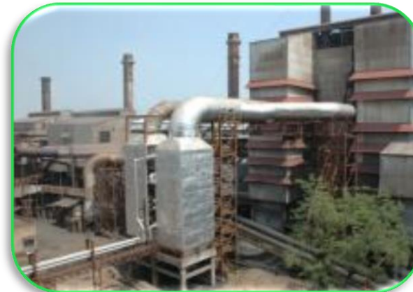
Waste Heat recovery system from furnace flue gas at Paloncha
